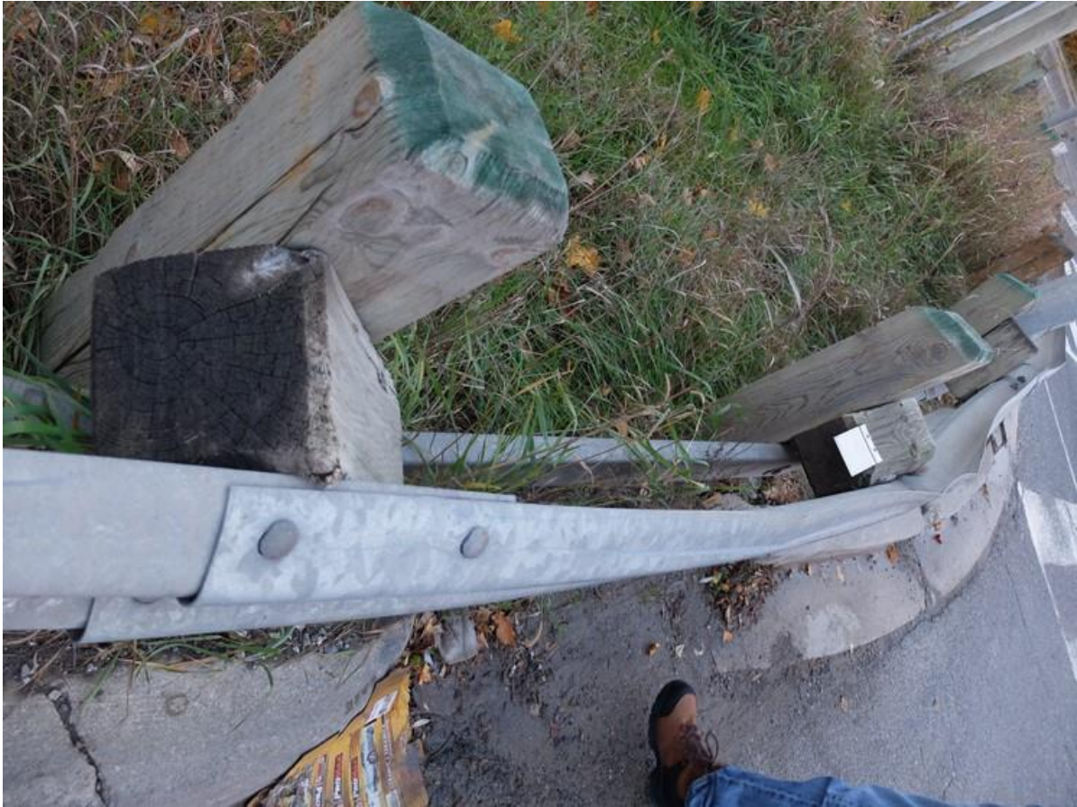
Figure 14: Damaged Guiderrail at Southeast Corner
