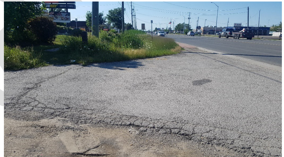
Image 4: View of disturbances associated with the asphalt roadway, concrete curb, paved shoulder, asphalt and gravel driveway, and ditching.
