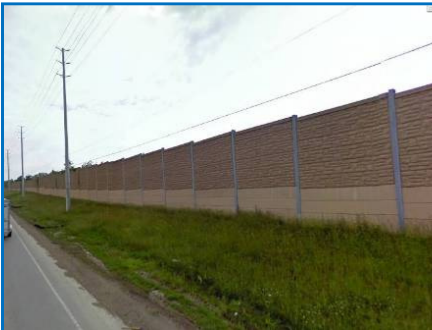
Figure 4 Noise Barrier along south side of Mayfield Road, west of Stonegate Drive.
