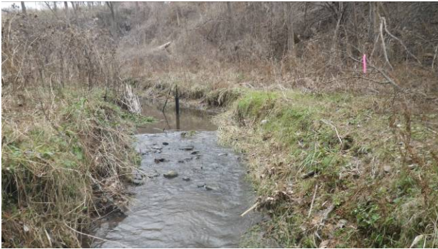
XS 6: View facing upstream. Bank erosion can be seen along both banks.
