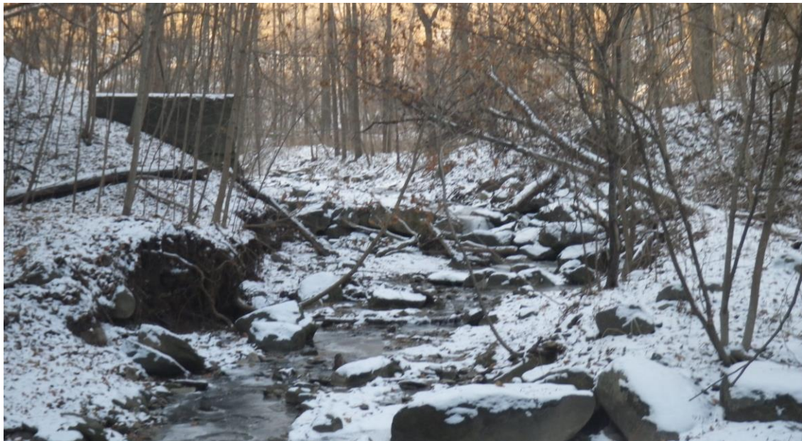
Figure 4.4: Photographs of existing fish barriers within Reach BV-A2, the perched culvert immediately DS of Bovaird Drive (top) and the relic weir approximately 60m DS of Bovaird Drive (bottom).
