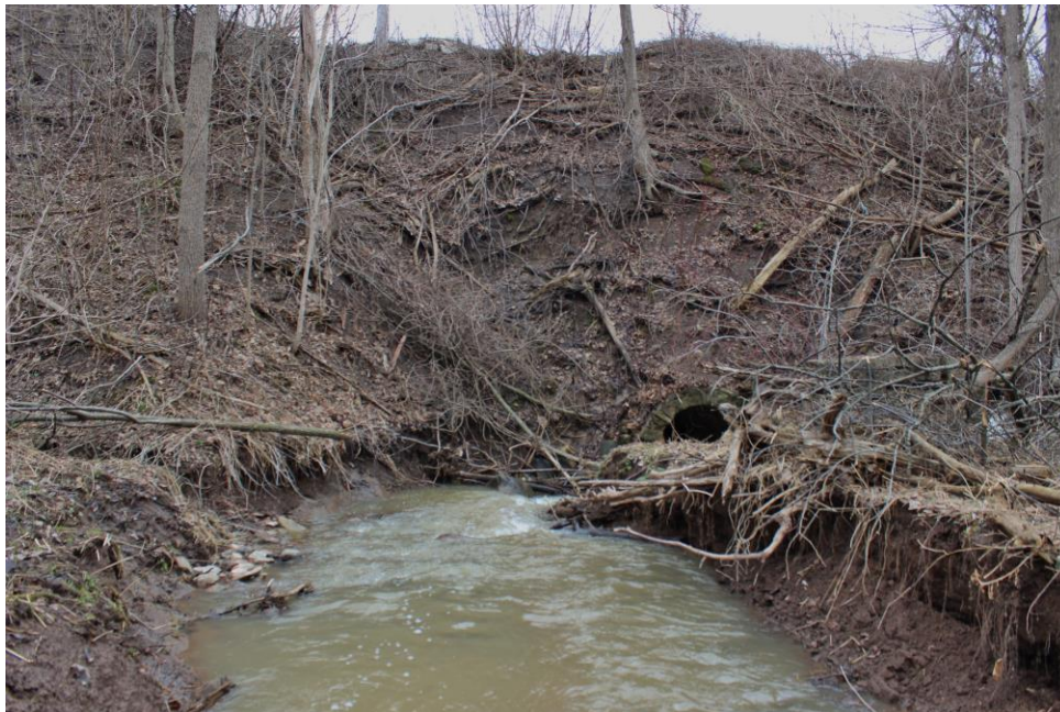
Figure 4.3: Photographs of existing culverts within Reach BV-A1, the small culvert approximately 250m US of Bovaird Drive (top) and the US (North) portion of the Bovaird Drive culvert (bottom).
