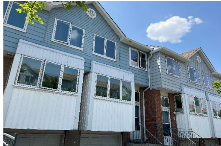
Creditbend Terrace windows replaced to improve energy efficiency and to maintain building condition for residents
